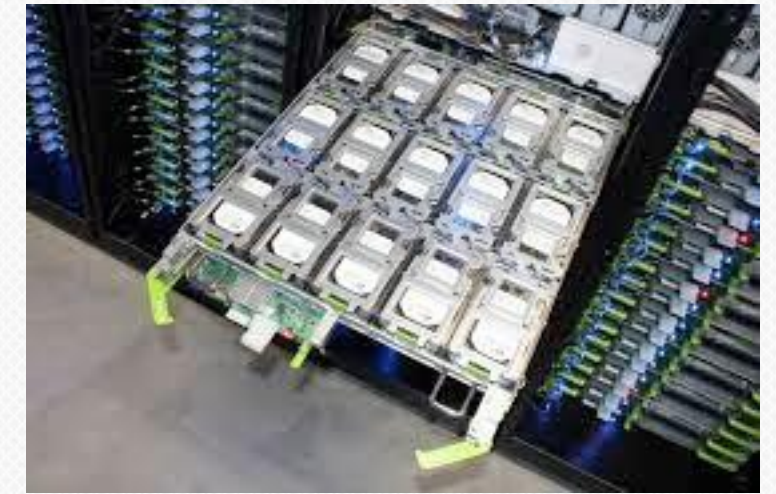
Facebook's Open Vault storage array. (Photo credit: Facebook)
